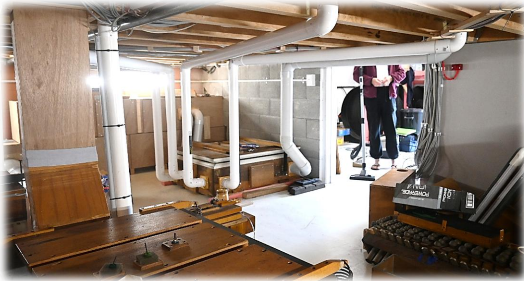
Wind lines and regulators fitted in the sub-chamber.
